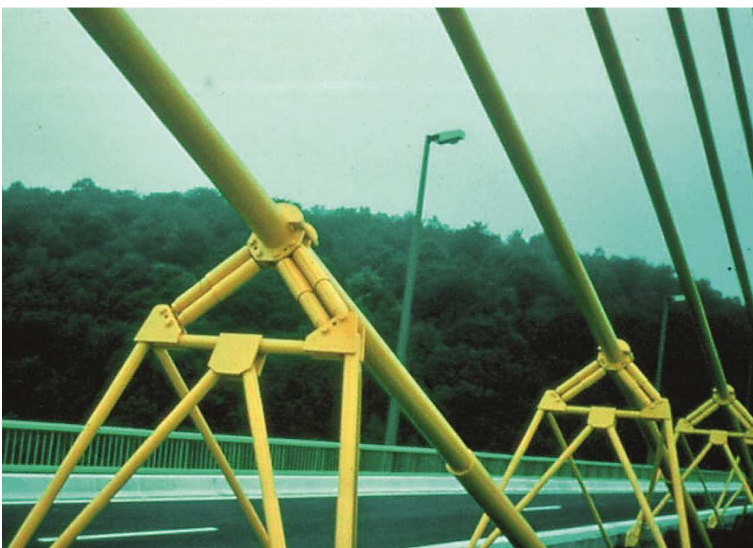
Figure 72: An early example of a discrete telescopic cable damper
