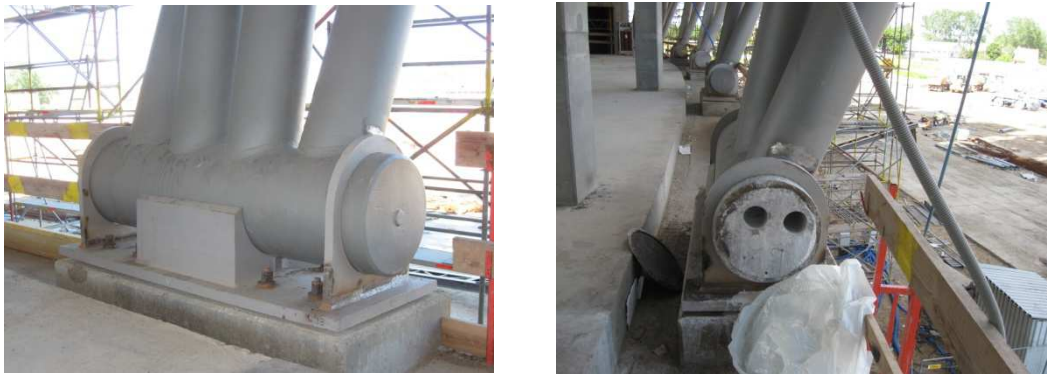
Fig.14 Support of the girder and the place where the samples were taken
